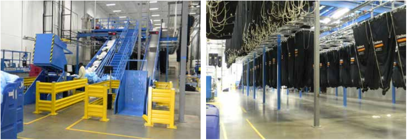
ABOVE: An automated system on a mezzanine may be used to sort items into batches of like items for washing; the system fills sling bags that are transported via rail to the wash area.
